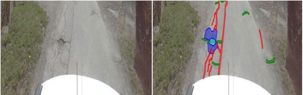
Display of annotated pothole together with longitudinal, transverse, and alligator cracks
