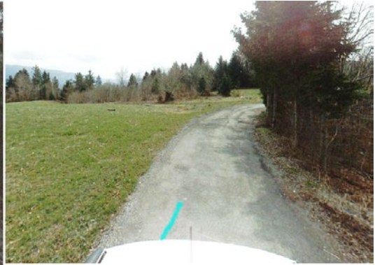
Road photo at station 2+702 showing pavement condition rated as 0
