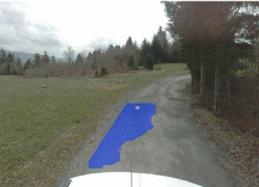
Road photo at station 2+707 showing pavement condition rated as 1
