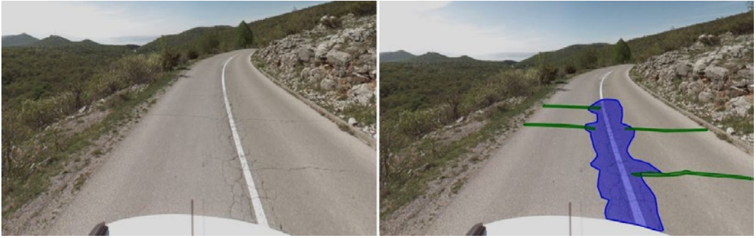
Display of annotated transverse cracks together with alligator cracking
