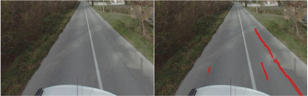
Display of annotated longitudinal cracks
