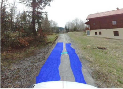
Road photo at station 2+764 showing pavement condition rated as 3
