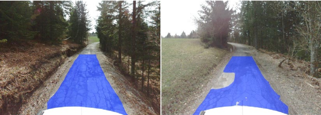
Road photo at station 2+500,00 showing pavement condition rated as 5
