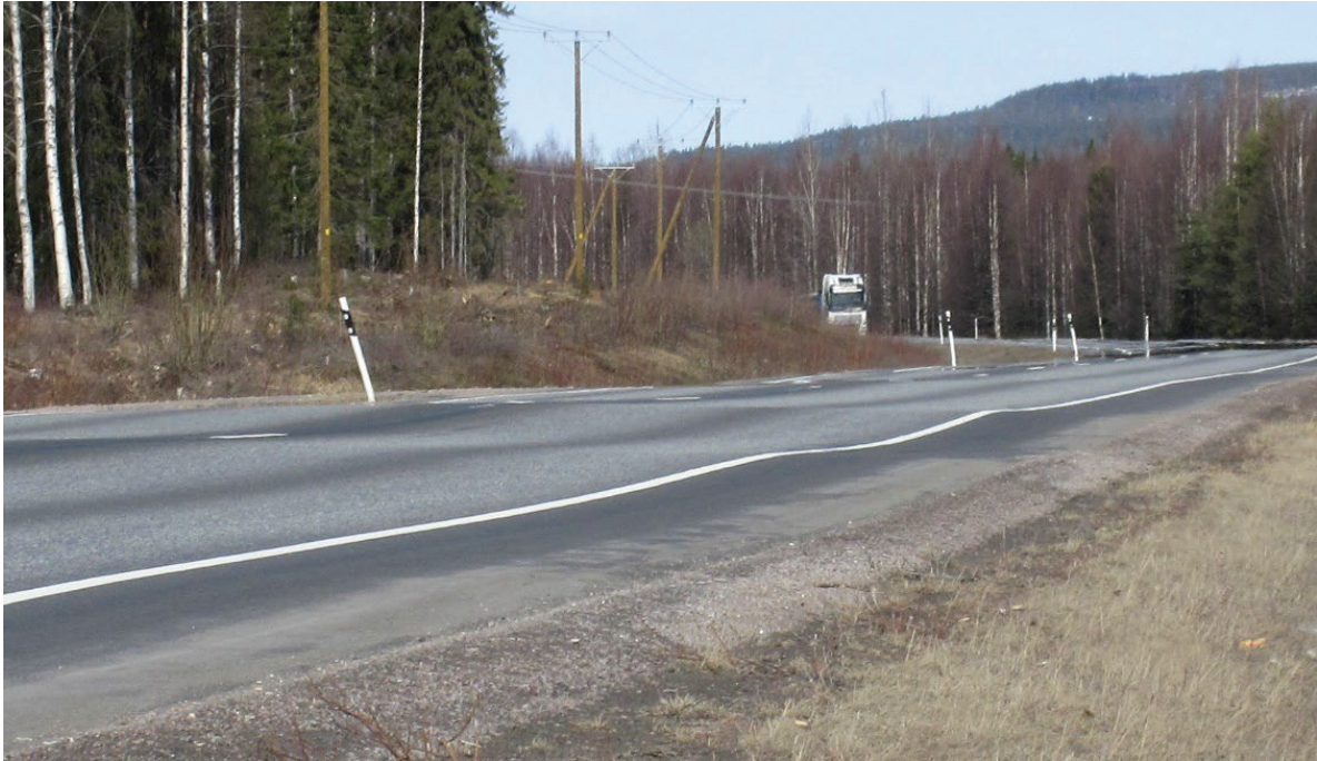
Fig. 11. Differential frost heave bump on Road 79 in Finnish Lapland in early May 2022
