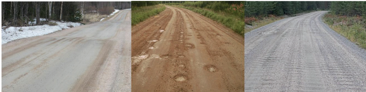
Fig. 7. Typical roughness problems of the gravel roads in Finland: bumps (left), potholes (middle) and washboarding (right).
